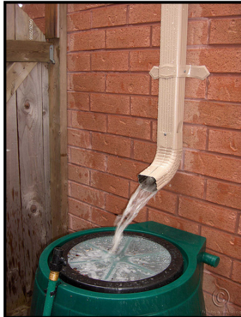
Figure. 4 Rainwater collection (through downpipes and sieves)
